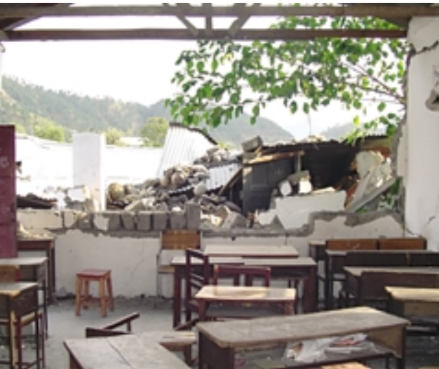
PAKISTAN: A school that was damaged by the South Asia earthquake.
